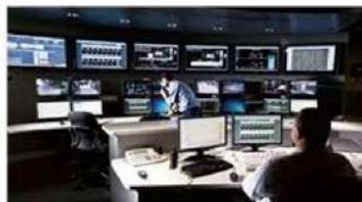
Command and control center
